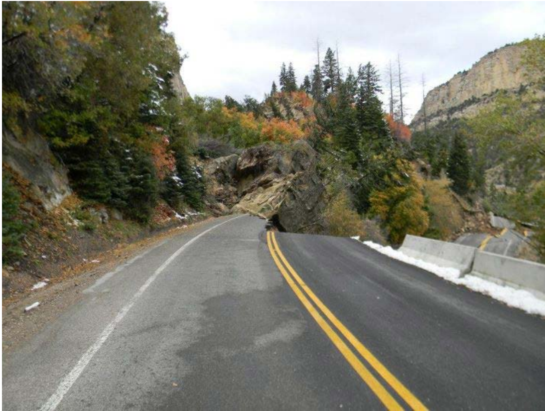
Figure C.20.1 Aftermath of Landslide on SR 14 (UDOT 2012)
